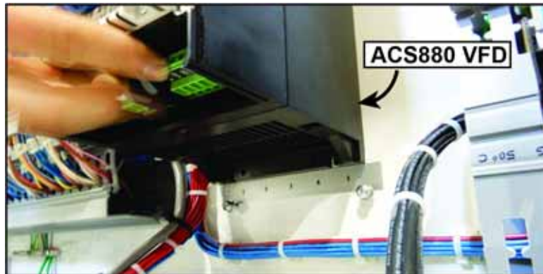
Figure 13: Placing VFD on a Ruler
