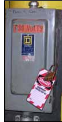
Figure 2: Lockout/tagout on the Power Source Panel
