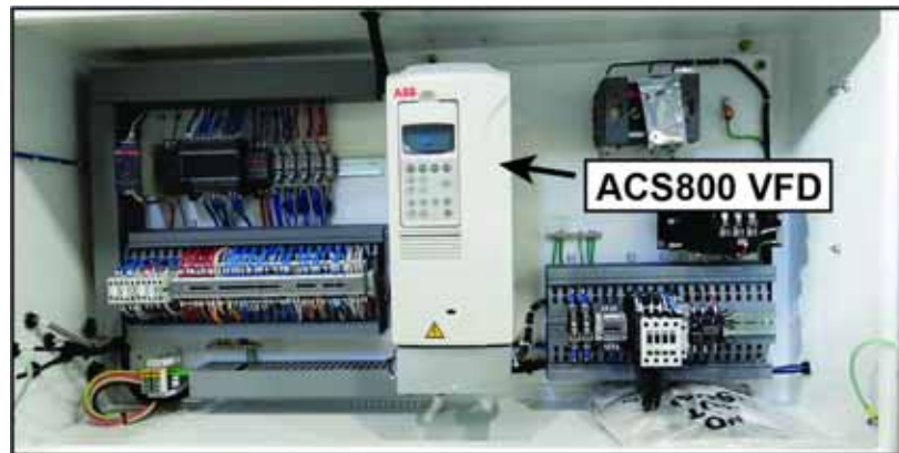
Figure 3: Location of the ACS800 VFD
