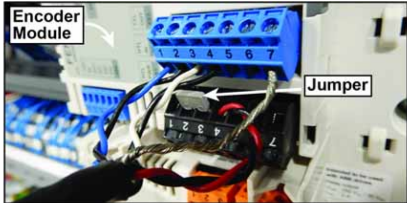
Figure 16: Encoder Module Wires
