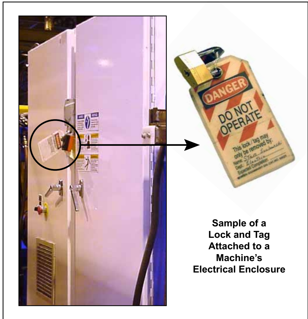
Figure 1: Lockout/Tagout on the Main Electrical Enclosure
