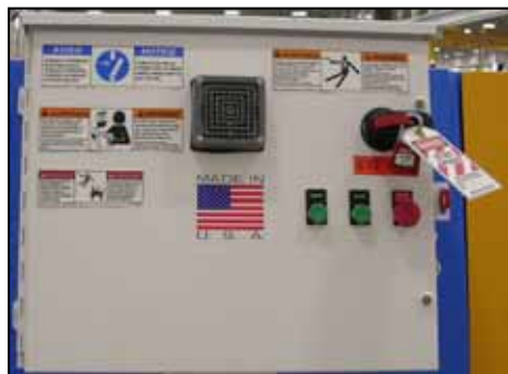
Figure 2: Lockout/Tagout on the Main Electrical Enclosure
