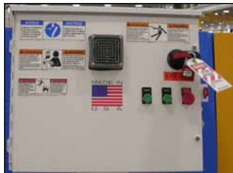
Figure 3: Lockout/Tagout on the Main Electrical Enclosure
