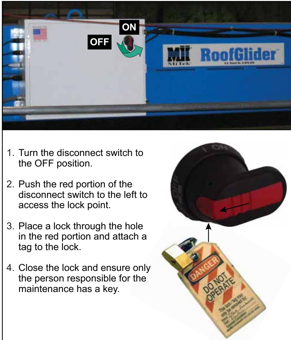
Figure 1: Lock and Tag Shown on Electrical Enclosure of a RoofGlider Press *
