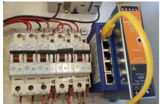
Figure 19: Yellow Cable Entering the Ethernet Switch
