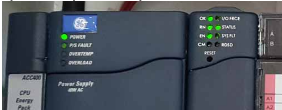
Figure 21: Checking PLC Indicator Lights
