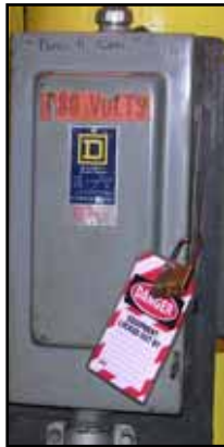
Figure 1: Lockout/Tagout on the Power Source Panel
