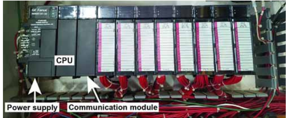
Figure 6: Locating the PLC
