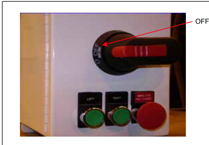
Figure 1: Power Off Switch
