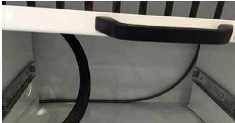
Figure 9: End-to-End Cable at Back of Enclosure
