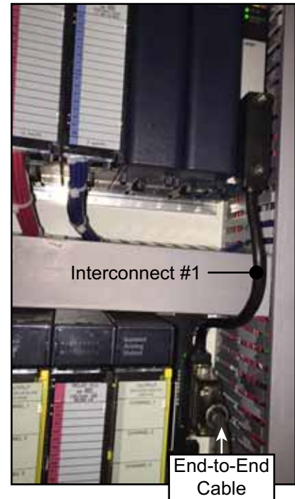
Figure 4: Cyber A/T, Rack 0 and Rack 1, Stationary End
