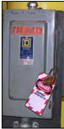
Figure 1: Lockout/Tagout on the Power Source Panel
