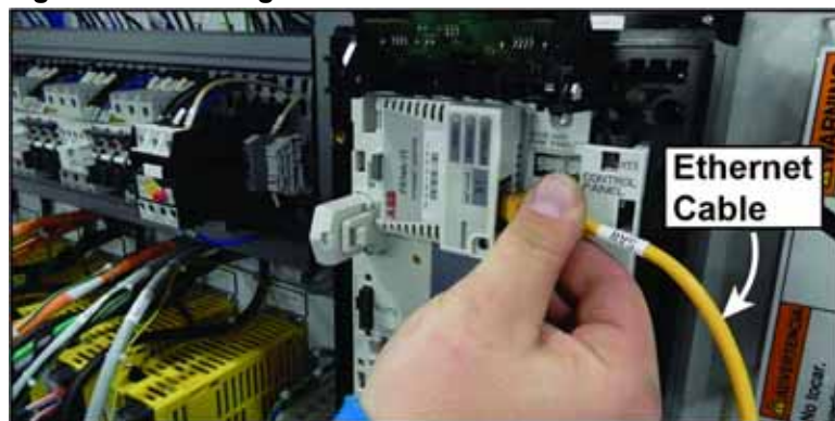
Figure 21: Inserting Ethernet Cable
