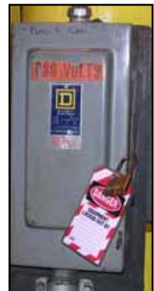
Figure 1: Lockout/Tagout on the Power Source Panel
