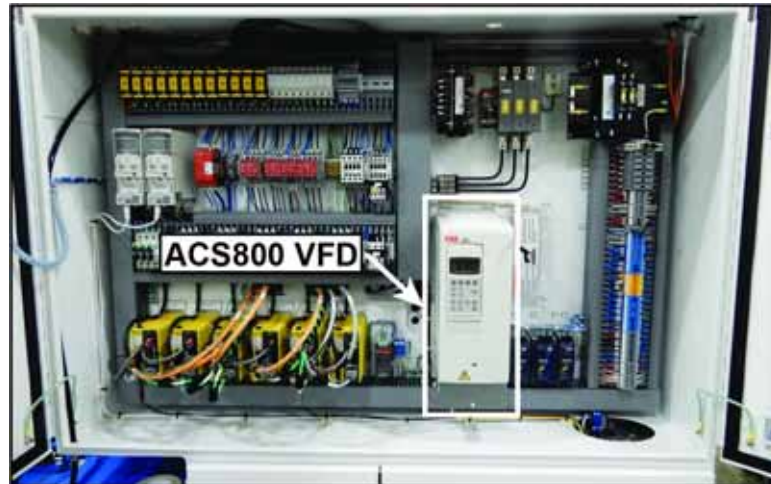
Figure 2: Obsolete ACS800 VFD
