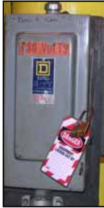
Figure 1: Lockout/Tagout on the Power Source Panel
